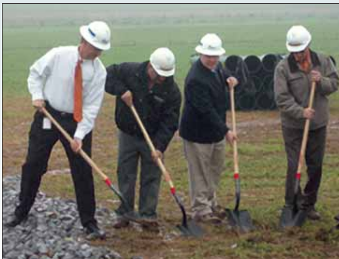
Senator Brubaker at the groundbreaking for the collaborative effort between Granger Energy and UGI to construct a nine-mile pipeline, which will be used to bring methane gas from the Conestoga Landfill to many industrial customers in the eastern Lancaster County area as a source of energy.
